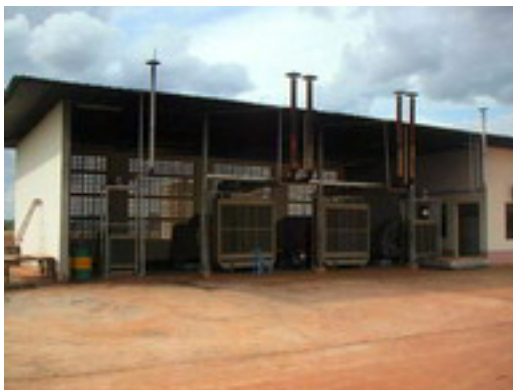
Picture 17: On-site generator sets
