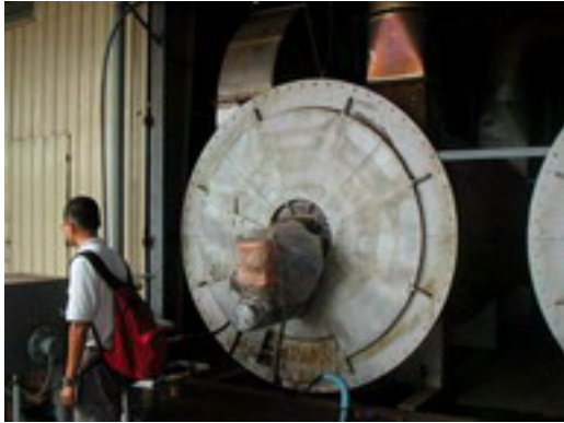
Picture 19: Steam boiler
